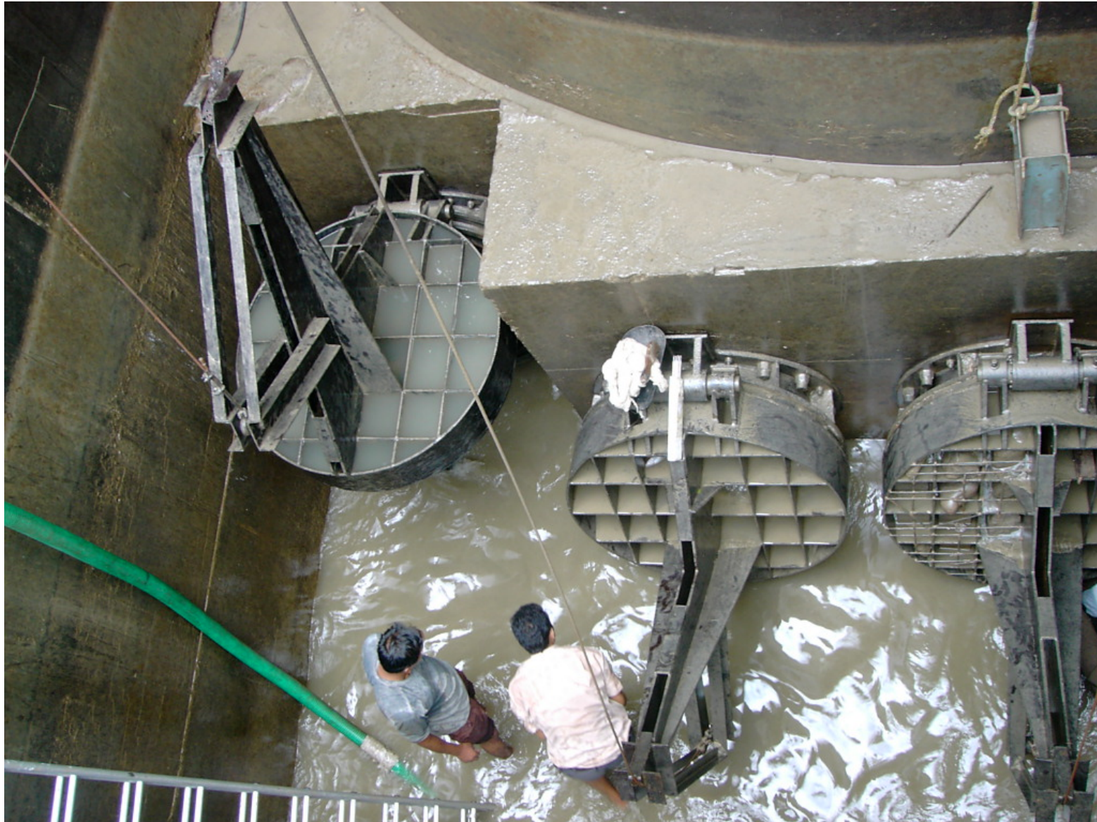
Jhimruk Power Plant, Nepal
