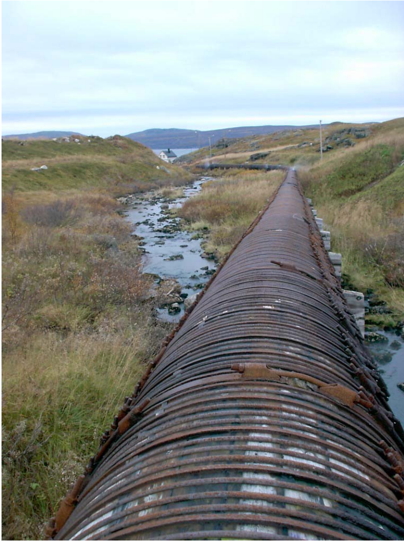
Breivikbotn Power Plant, Norway
