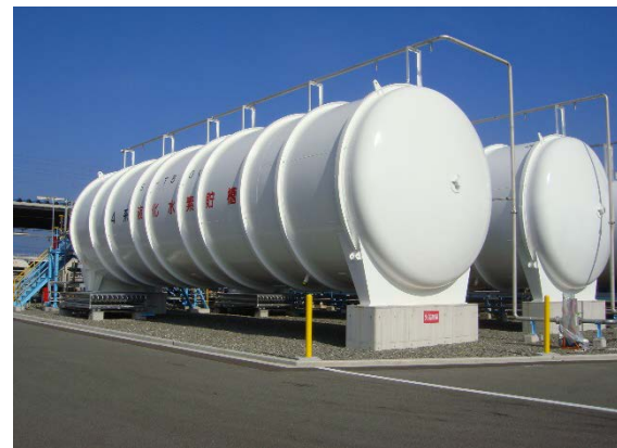
Liquid hydrogen storage tank
