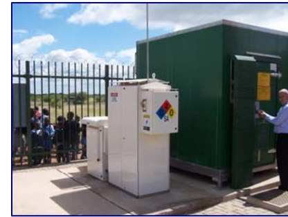
A PlugPower GasCore Fuel System in South Africa provides back-up power for telecommunications.
