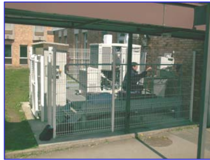
A PlugPower natural gas fuelled CHP unit powers a greenhouse in Nancy, France.
