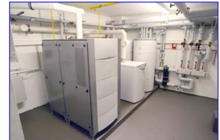
A Vaillant fuel cell heating appliance, Oldenburg, Germany.
