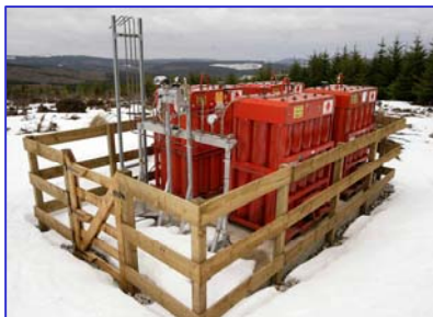
A PlugPower GasCore Fuel System provides power to a telecommunication mast in Scotland, United Kingdom.
