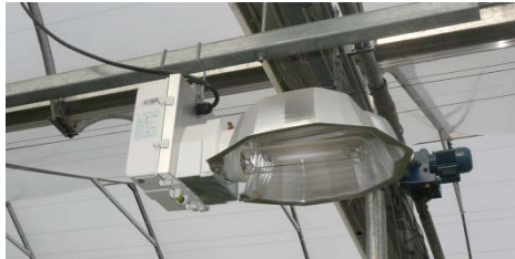
Figure 9. High Intensity Discharge (HID) luminaire in a greenhouse.
