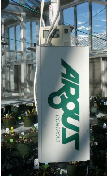
Figure 10. Aspirated box in a greenhouse. A fan draws air from the bottom of the box over the sensors.
