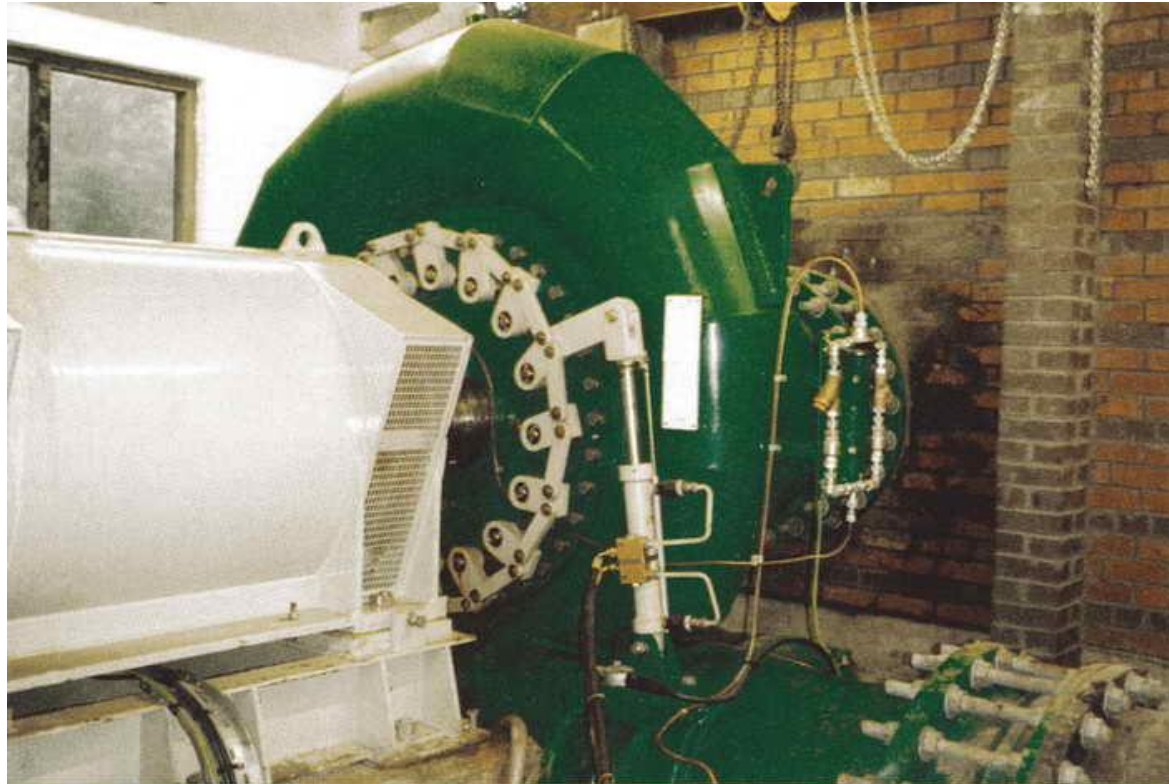
Figure 5.17 The 450 kW horizontal-axis Francis turbine of a small-scale plant in Scotland, commissioned in 1993. The inflow (at lower right) is 2.1 \text{ m}^3 \text{ s}^{-1} at a head of 25 m. The turbine, rotating at 750 rpm, drives the generator whose casing can be seen on the left
