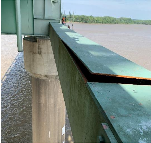
c. Cracked longitudinal fillet weld connecting top plate to inboard side plate (view looking west).
