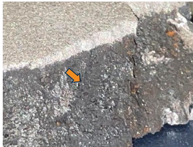
Figure 34. Previous arrest mark (arrow away from the crack tip).
