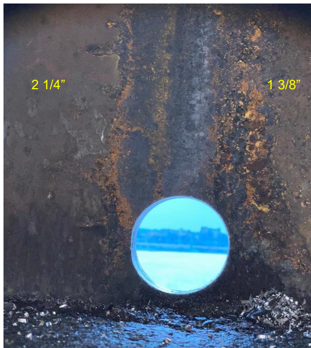
Figure 15. View from inside tie showing core sample removed from groove weld.
