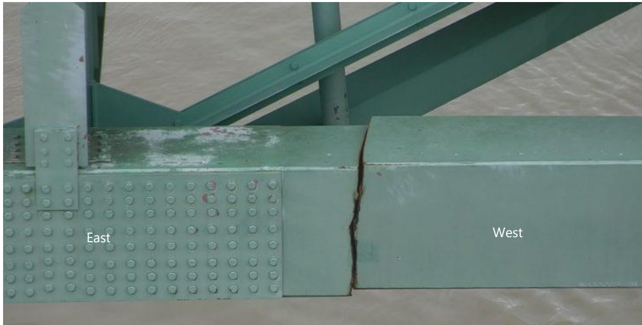
Figure 1. Annotated photo of partial tie girder fracture identified in May 2021 (photo courtesy of TDOT).
