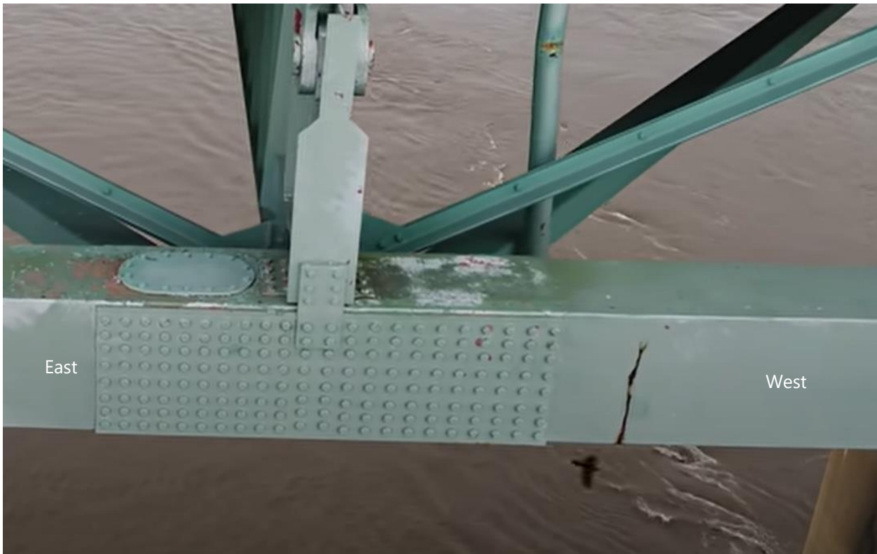
Figure 8. An annotated screen-capture of the crack found by drone video footage from the May 2019 MBI inspection.
