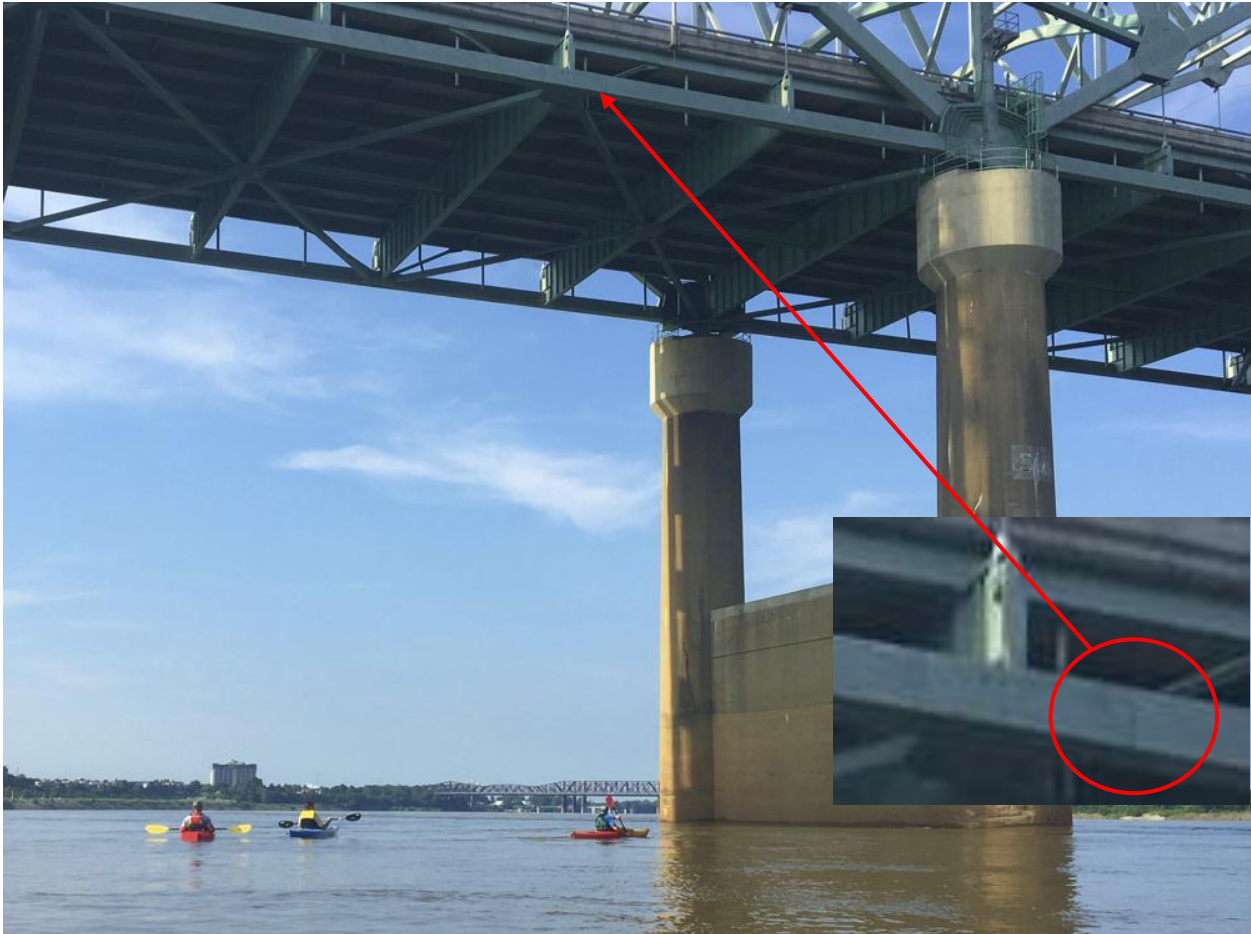
Figure 9. 2016 crack-like indication in tie girder (photo from Barry W. Moore via AP).
