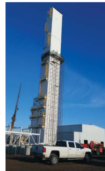
Construction gets underway on Air Separation Plant distillation column at Cristal Global jobsite, where Local 673 members are working.
