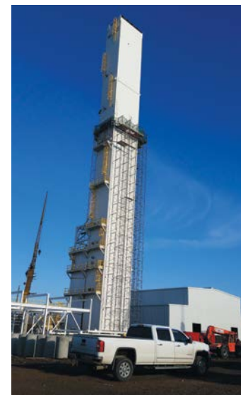
Construction gets underway on Air Separation Plant distillation column at Cristal Global jobsite, where Local 673 members are working.
