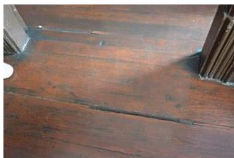
Figure 12 - Wood wear on stairs
