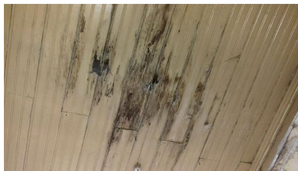
Figure 14 - Consequences of dampness in ceiling
