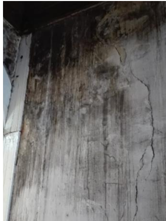
Figure 10 - Dampness, cracks and mould in an interior wall
