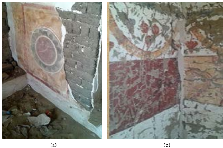
Figure 2. The critical state of conservation of painted surface at the necropolis of Tuna el-Gebel: (a) fallen, losing and separation of painted layer; (b) extensive network of micro-cracks.
