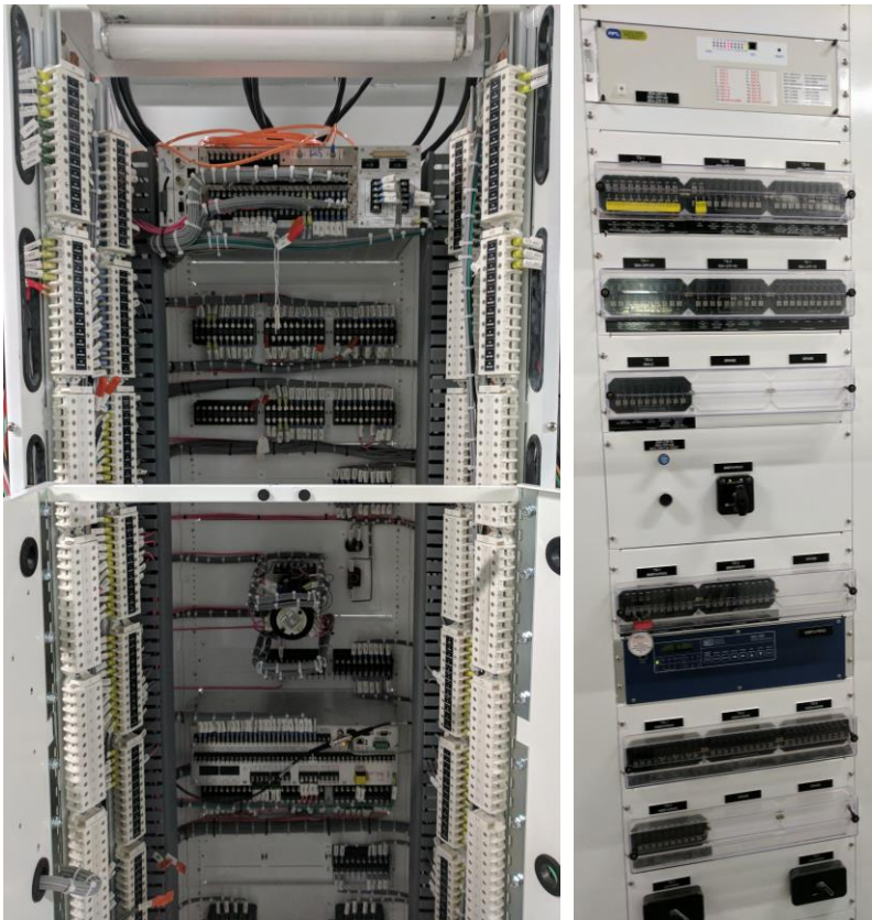
Example of a recently constructed control panel
