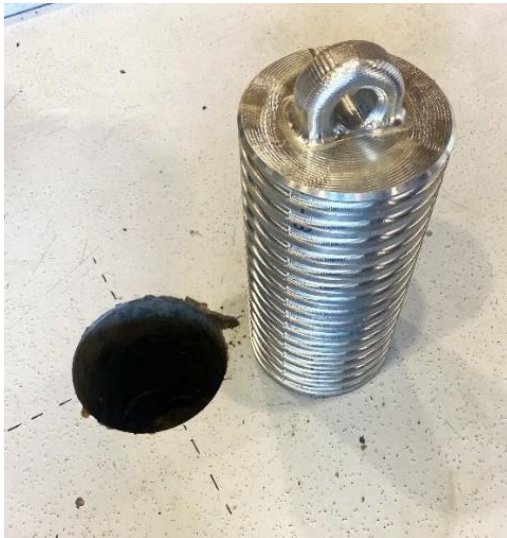
Figure 15: Concrete core drilled out of hangar slab to allow the ILDFA tie down point to be chemically anchored.
