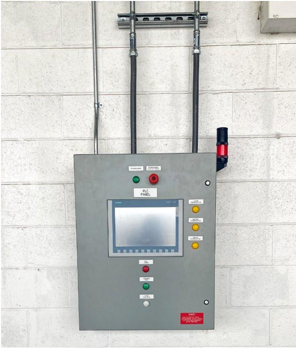
Figure 21: ILDFA Control Panel mounted on the interior hangar wall.
