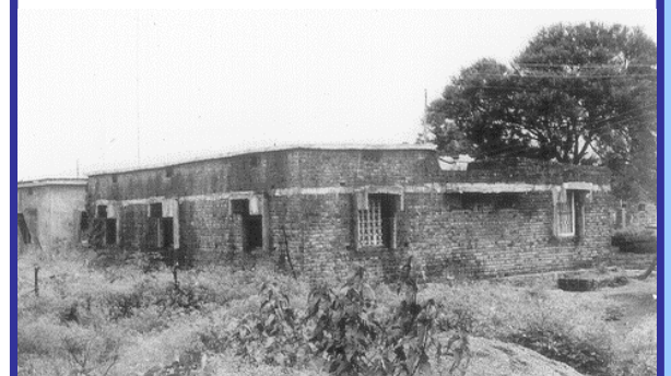
(b) A building with horizontal lintel band in Killari village: no damage
