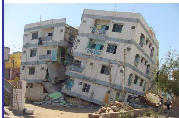
(b) Collapse of reinforced concrete columns (and building) during 2001 Bhuj (India) earthquake
