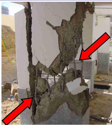
Figure 3: Diagonal cracks in columns jeopardize vertical load carrying capacity of buildings - unacceptable damage.
