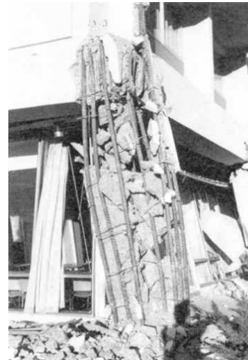
(b) Brittle failure of a reinforced concrete column
