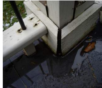
Top mounted guard posts should be avoided
