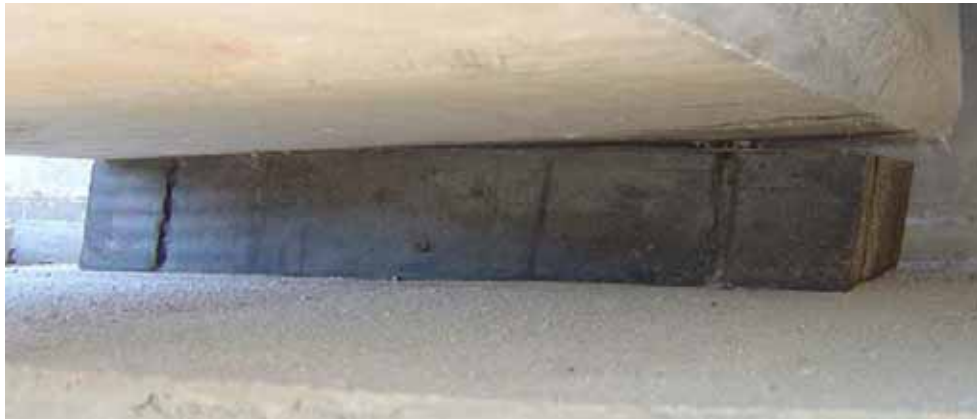
Figure 2.15: Lift-off of Fascia Girder from Bearing Pad
