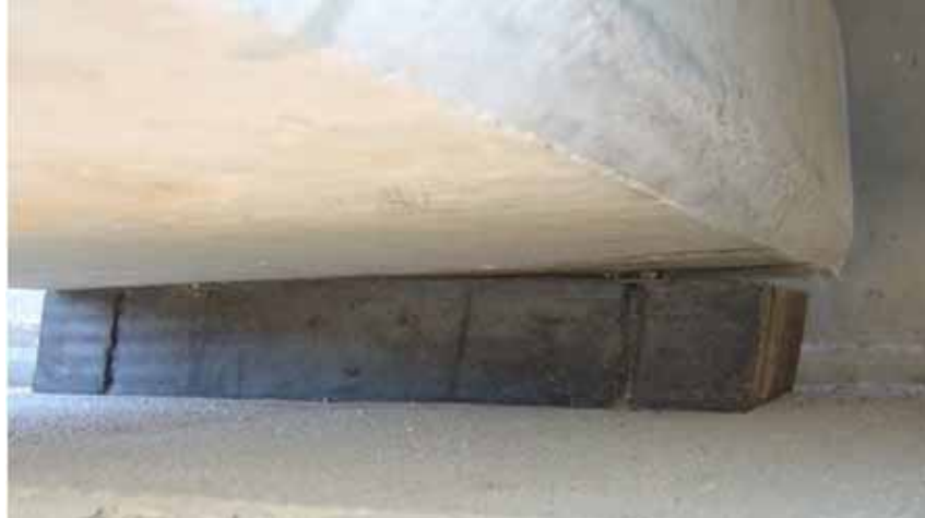
Figure 6.2: Lift-off of Fascia Beam at Hutto Concrete Bridge
