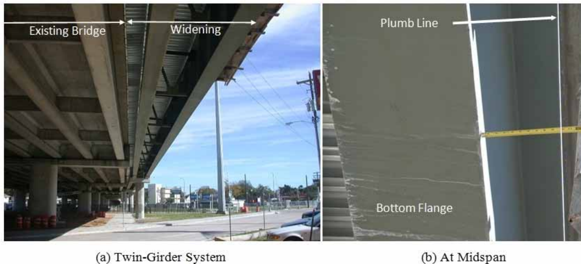
Figure 2.13: Twin-Girder Widening with Excessive Girder Rotation
