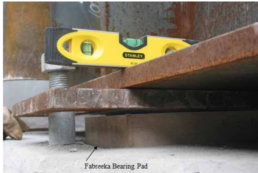
Figure 4.19: Fabreeka Bearing Pad in Place
