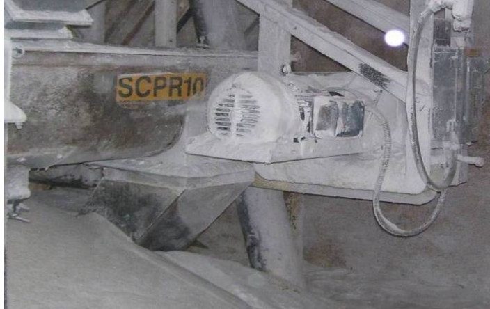
Figure 19. Motor cooling fins and fan guard covered with sugar dust; large piles of sugar cover the floor (Imperial Sugar photo)
