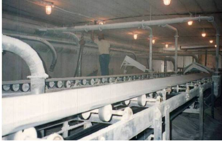
Figure 8. Granulated sugar steel conveyor belts above the silos, circa 1990. Heavy dust accumulation on conduit and spilled sugar on the floor (Imperial Sugar photo)
