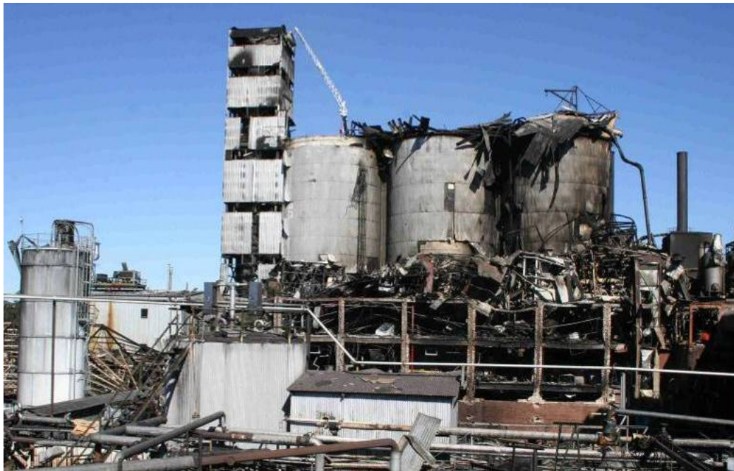
Figure 1. West bucket elevator tower; silos 3, 2, and 1; and south packing building destroyed by the February 7, 2008, sugar dust explosions and fires
