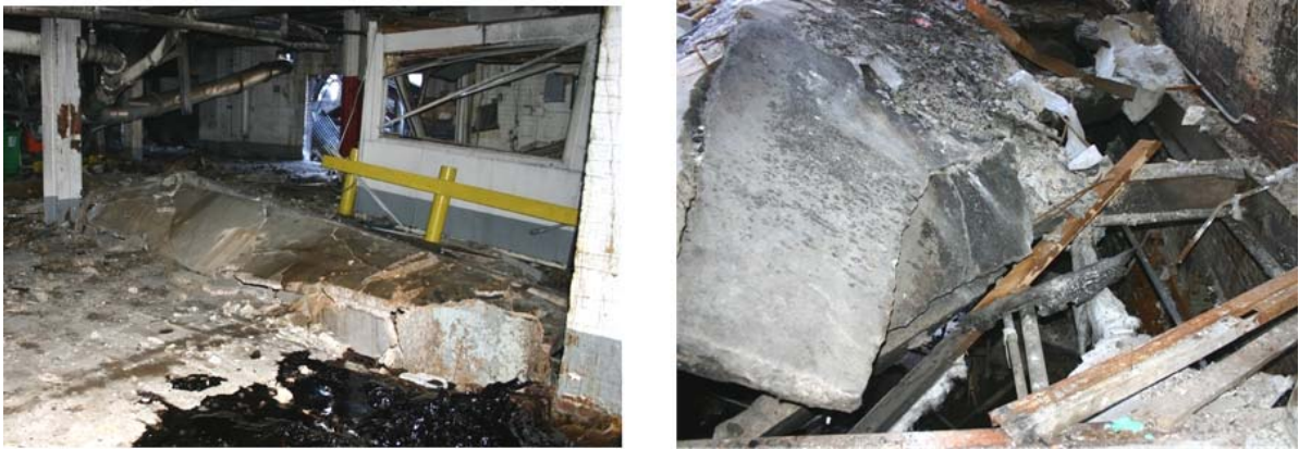
Figure 18. Three-inch thick concrete floor slabs lifted off the steel supports by the explosion pressure waves
