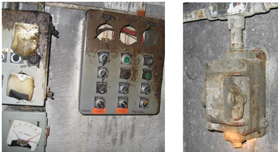
Figure 22. Non-dust rated and rated electrical devices in the silo tunnel
