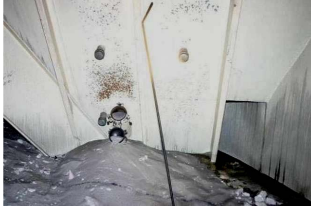
Figure 16. Access port inside the pantleg room and steel rod used to break sugar lumps in the sugar outlet on silo floor
