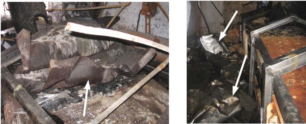
Figure 13. Steel belt covers (arrows) crumpled from an initial dust explosion inside the steel belt enclosure (steel frame structure, right photo)
