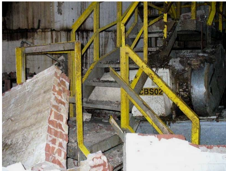
Figure 15. South stairwell brick walls blown into the packing building
