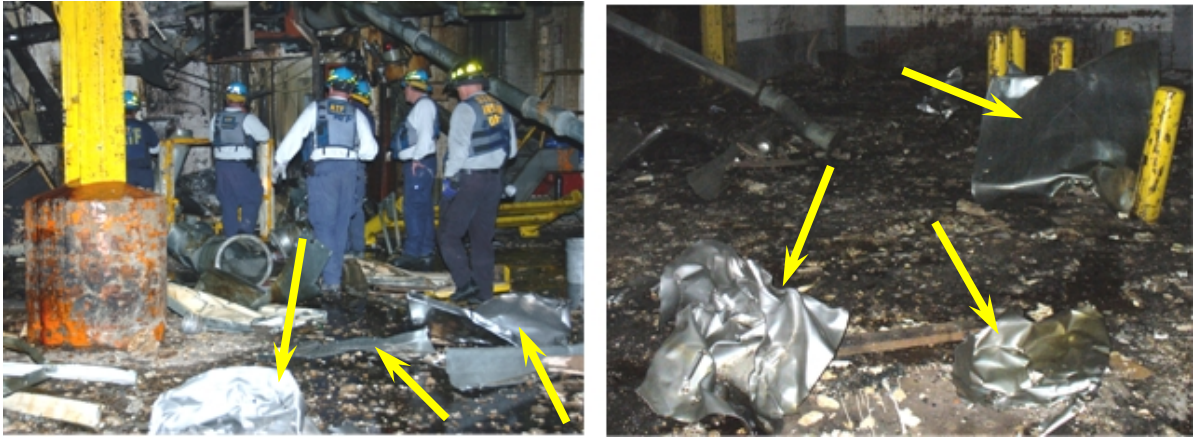
Figure 14. Stainless steel cover panels (arrows) blown off the steel belt enclosure and out of the tunnel into the packing building
