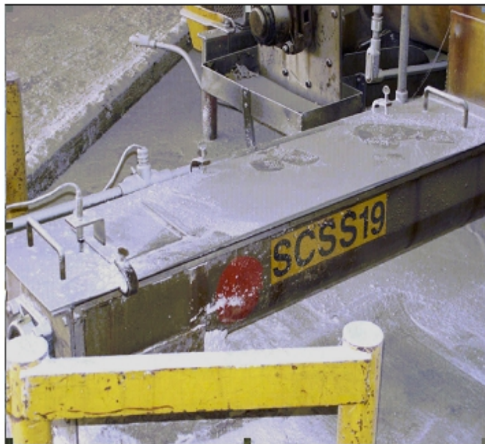
Figure 23. Sugar and dust accumulation on a screw conveyor in the south packing building fourth floor near silo 1 (Imperial Sugar photo)
