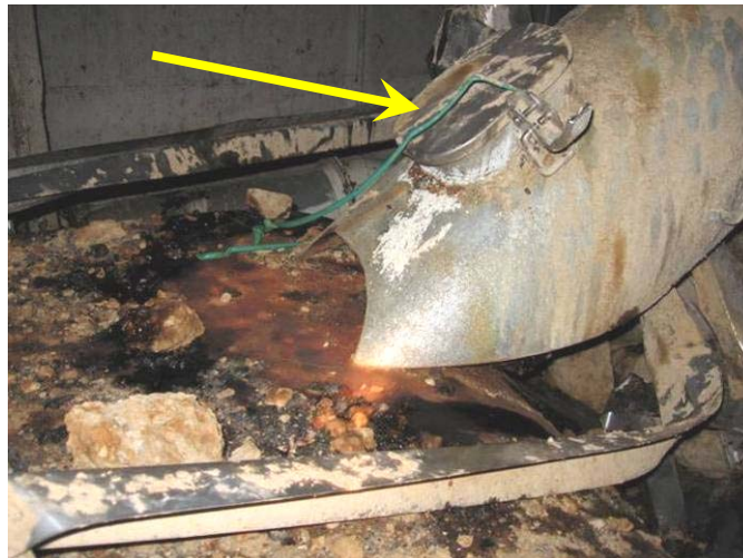
Figure 17. Limited clearance between sugar discharge chute and the steel belt would sometimes be blocked by large sugar lumps; lump-clearing access port (arrow) is on top of the chute
