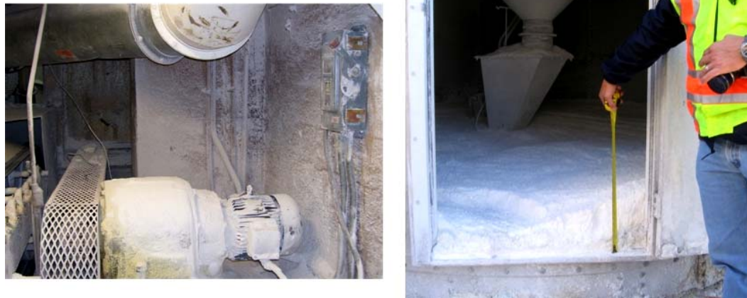
Figure 21. Left: Sugar dust accumulation on steel belt drive motor in silo tunnel (Imperial Sugar Co. photo, Oct. 2006). Right: Cornstarch spilled under cornstarch silo (March 2008).
