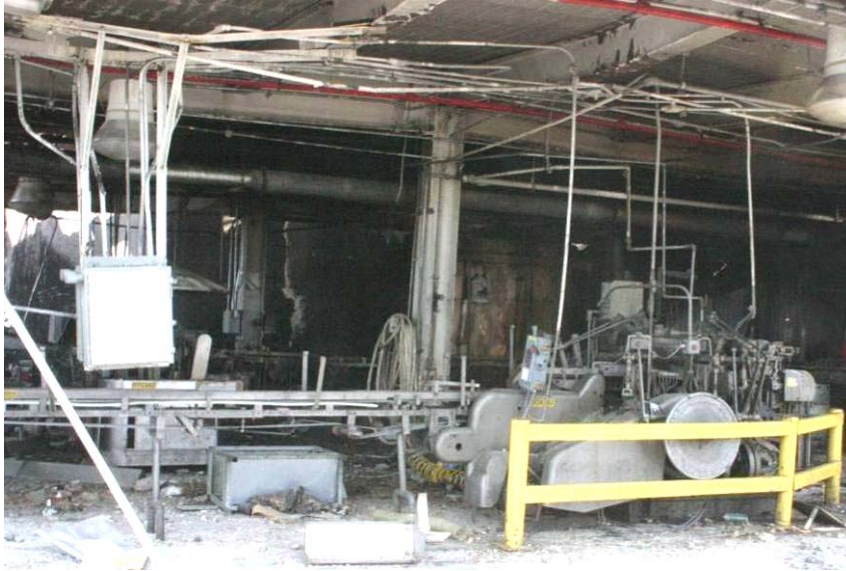
Figure 20. Packaging equipment hindered evacuation in the darkened building
