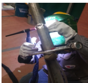
1. 6G pipe welding certification test The welding was done with 6G pipe fixed at a 45° angle to the base position.
