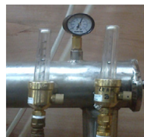
4. Premixed gas cylinder The shielding and purging gas used was Argon+2% nitrogen, supplied from a premixed gas cylinder.
