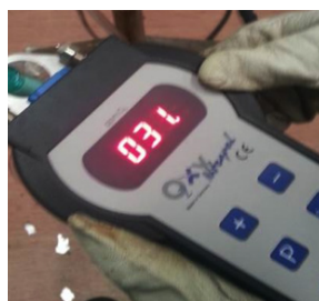
3. Calibrated oxygen monitor With the help of a calibrated oxygen monitor, the oxygen level was kept below 100 ppm on the root side during welding.
