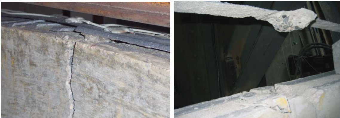
Figure 74. Failure mode of beam 2 (left) and beam 2D (right).
