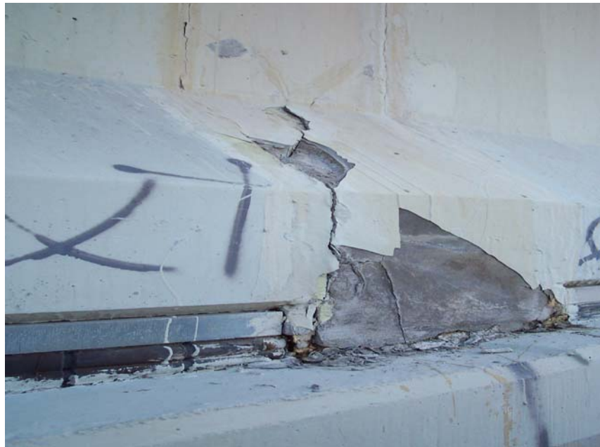
Figure 23. Diaphragm crack at fascia beam (Rt. 1&9, Newark).
