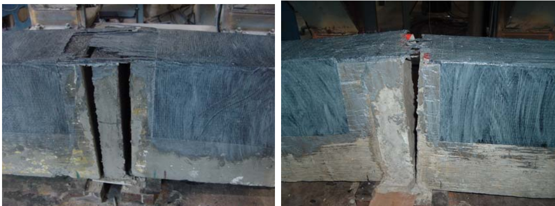
Figure 89. CFRP rupture of beams 17 (left) and 18 (right).
