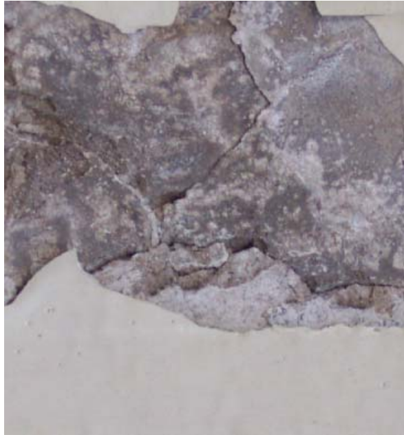
Figure 25. A close-up of the crushed concrete at fascia beam (Rt. 1&9, Newark).
