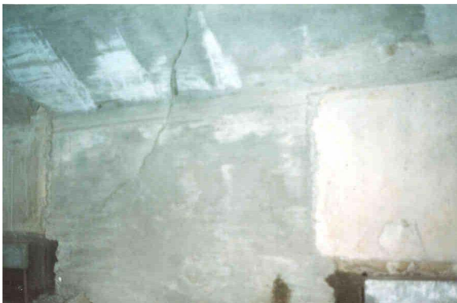
Figure 24. Typical diaphragm crack at inner beams (Rt. 1&9, Newark).
