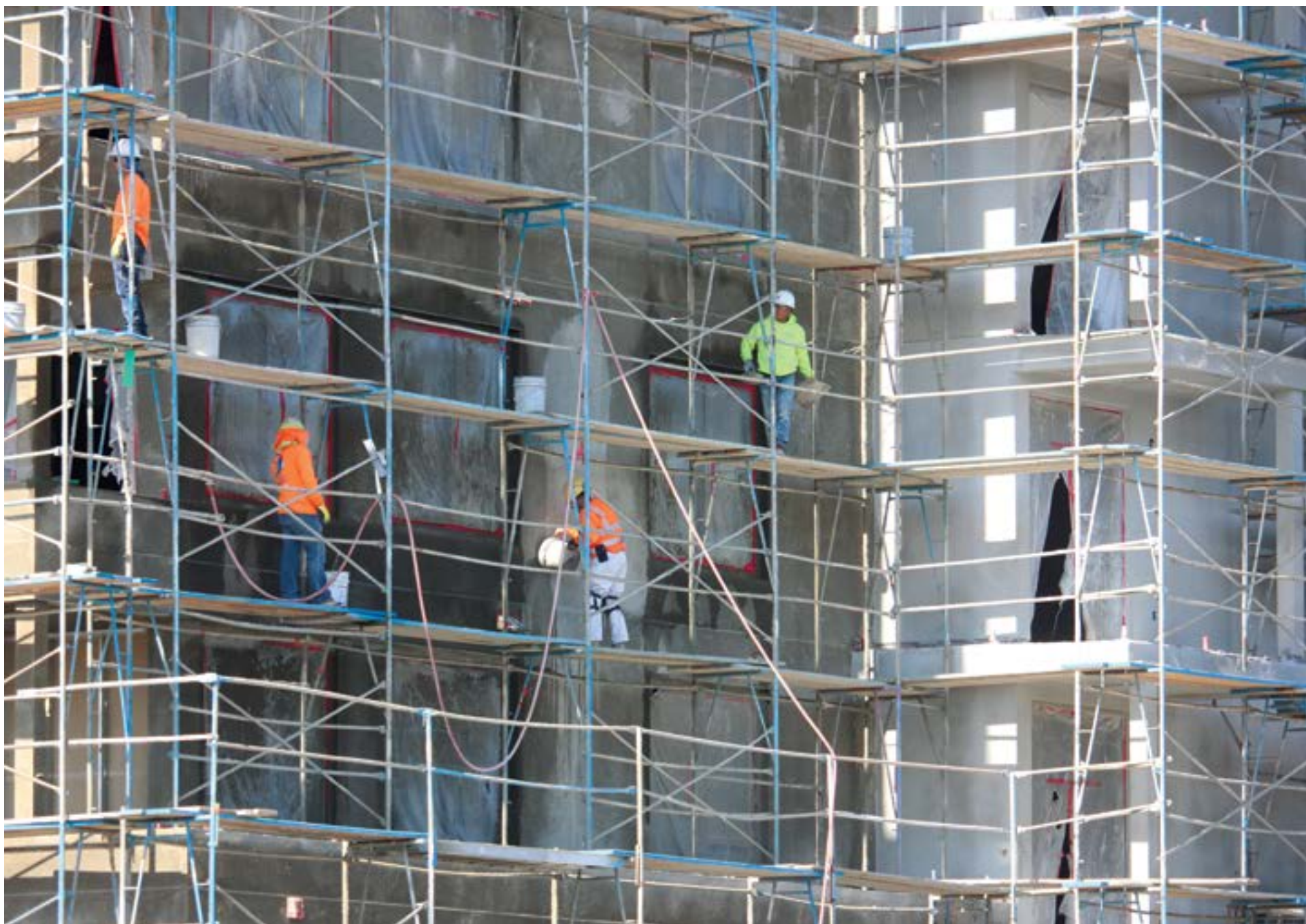
Crews work on the exterior of Union South Bay, located across the street from Carson City Hall. (Photograph by Brandon Richardson)
