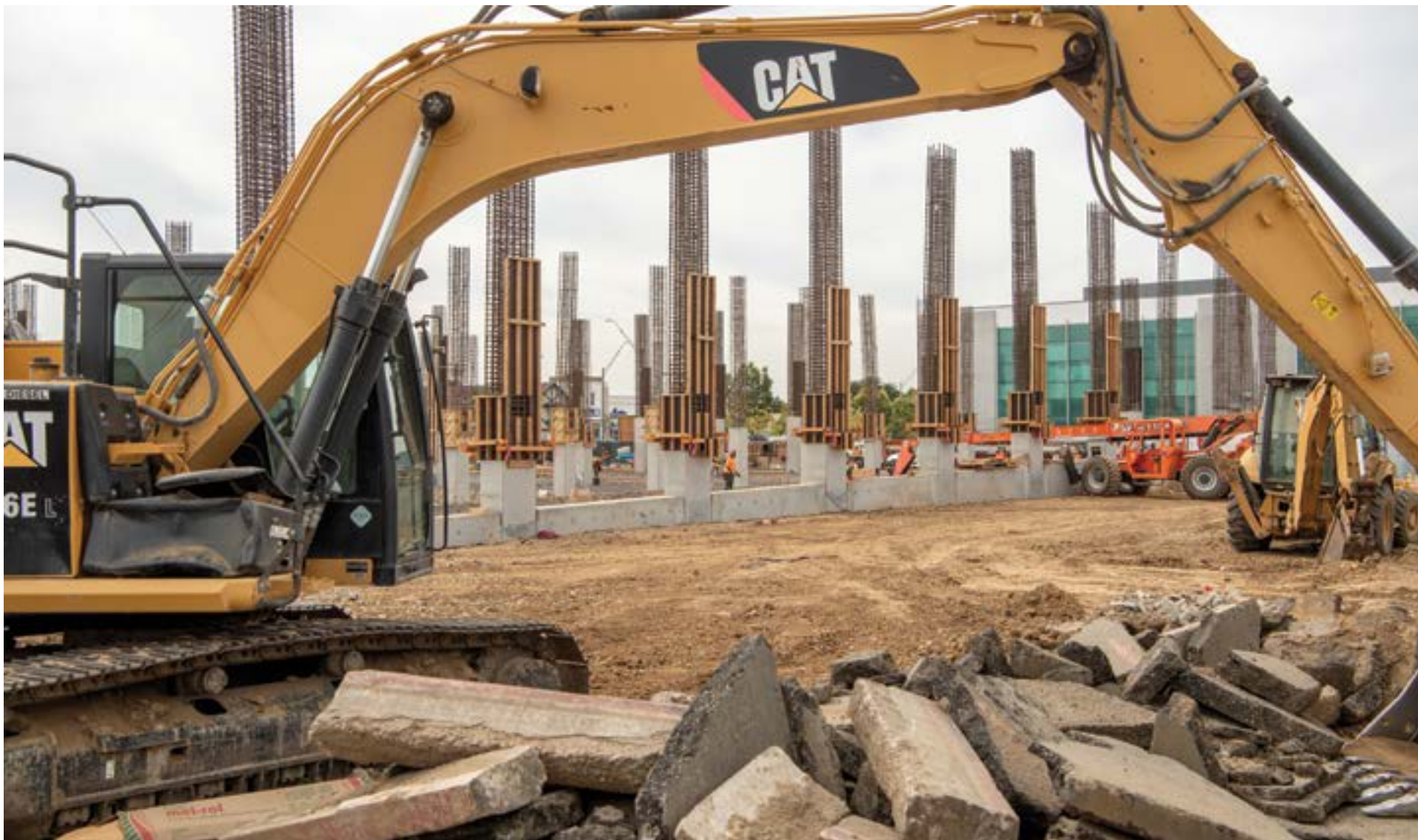
Construction is underway on an $18.4 million, 530-stall parking structure at Long City College's Pacific Coast Campus. The project is being paid for using Measure LB bond funds approved by voters in 2016. (Photograph by Thomas Cordova)
