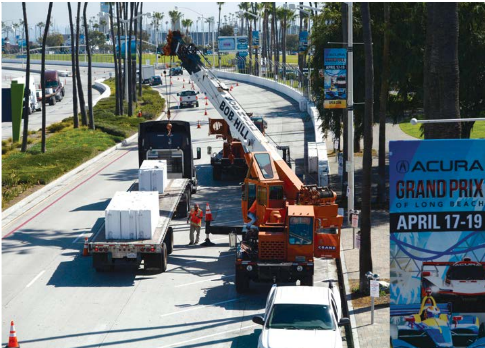
Crews work on the newly installed barriers along Shoreline Drive in Downtown for the Acura Grand Prix of Long Beach.
