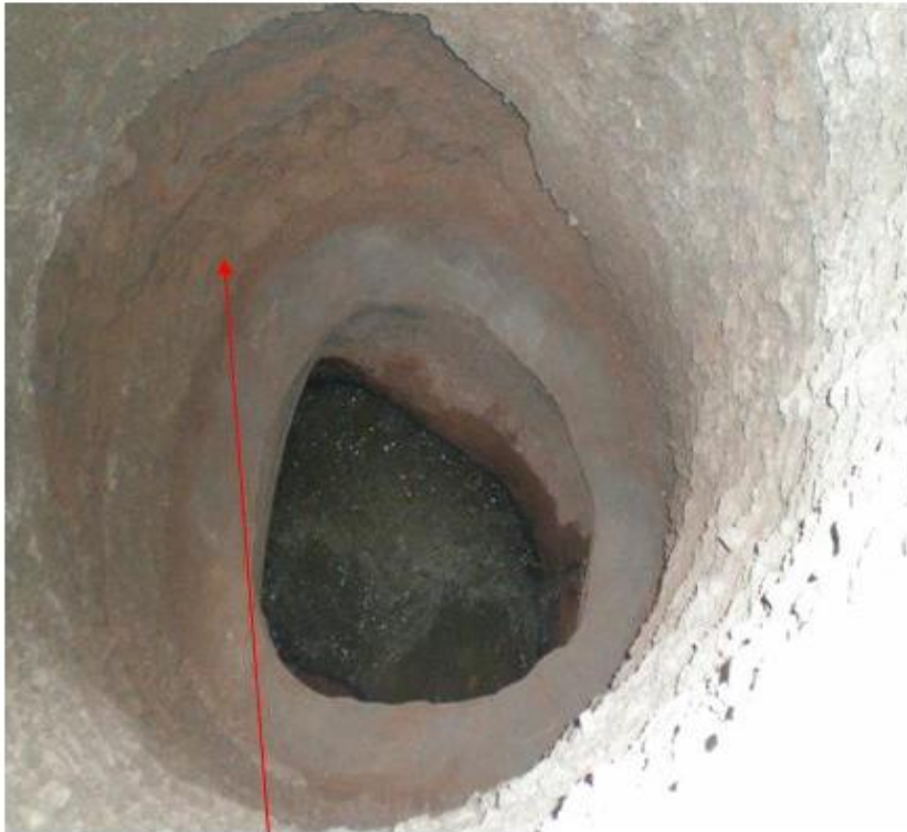
Missing barrel section
