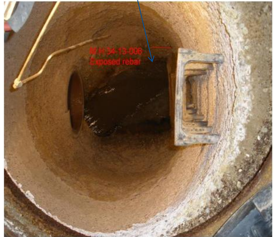
Exposed , Sharp Rebar
