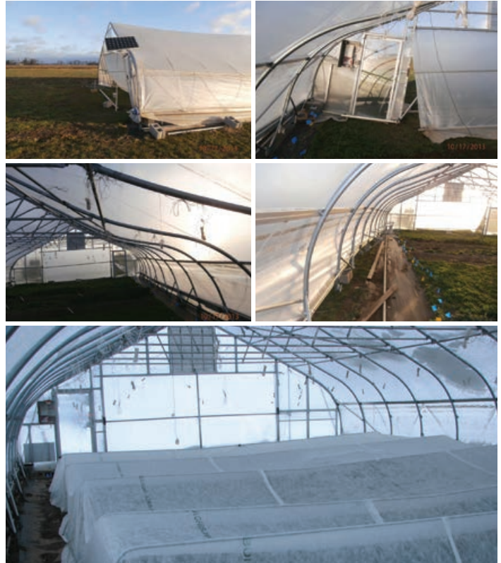
Wind can seriously damage high tunnels. These photos show a high tunnel with bent metal structures and posts pulled out of the ground. A nearby weather station recorded sustained winds of more than 20 mph and gusts of more than 50 mph. After the damage, the owner installed a vertical post to reinforce the wide curtain end wall (you can see this in the center of the bottom photo). The post also helps prevent the end wall from billowing inward during high wind.
