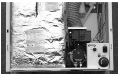
Figure 4-1: Boiler front panel open
