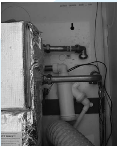
Figure 6-2: Condensate trap location in-situ
