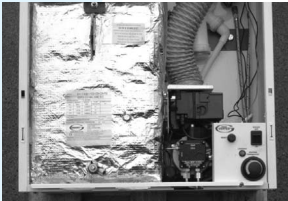
Figure 9-1: Boiler lower front panel in down position
