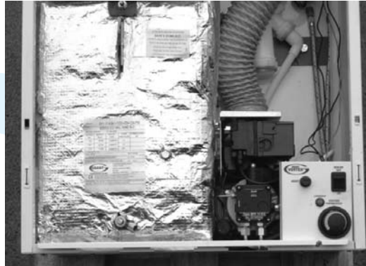
Figure 1-1: Boiler lower front panel in down position
