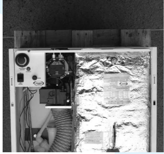
Figure 1: Boiler lower front panel in down position
