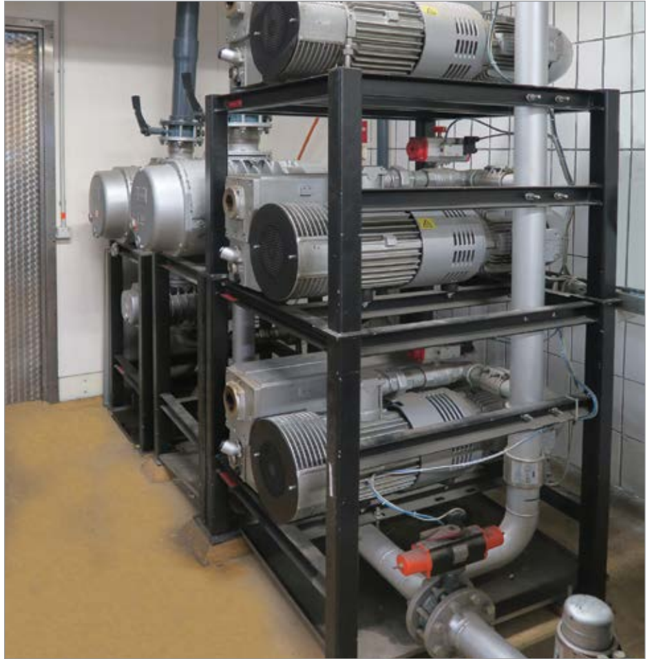
Shown is the central vacuum system at Peter Mattfeld & Sohn's operation.
