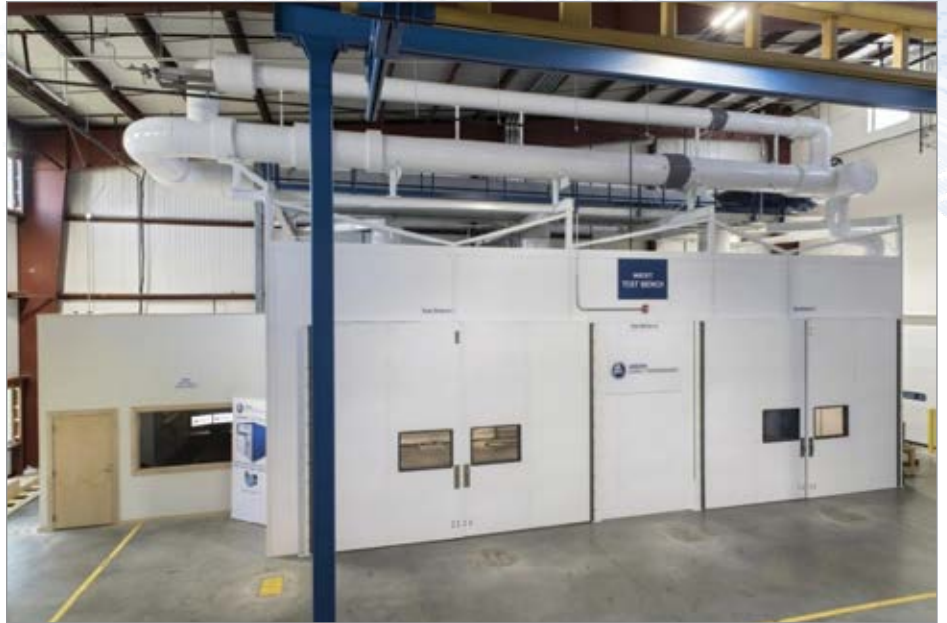
The ASME PTC 13 conforming factory test facility at the Aerzen Coatesville, Pennsylvania, facility.
