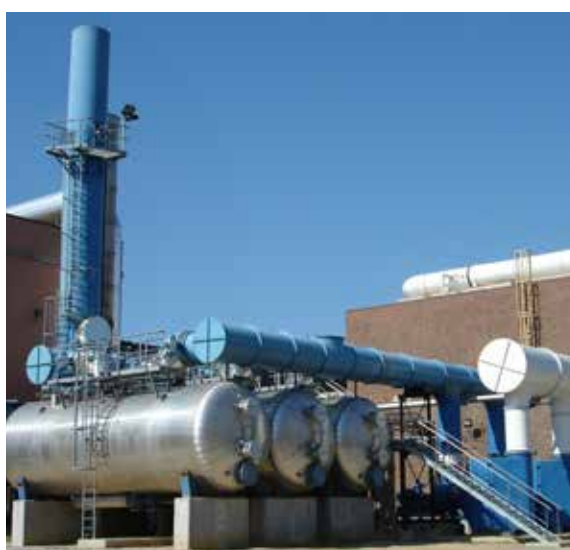
Large carbon adsorption solvent recovery system
