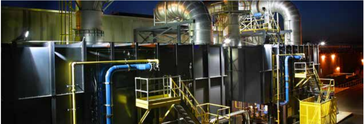
Regenerative thermal oxidizers with switch valve
