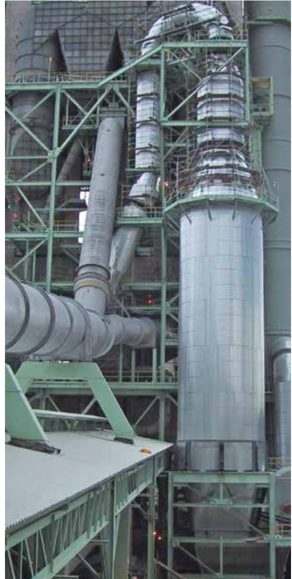
Evaporative gas cooling system in cement plant
