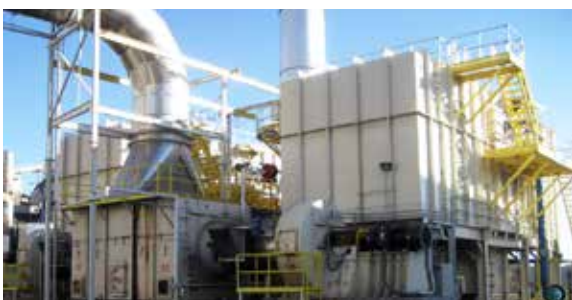
RTO with switch valve
