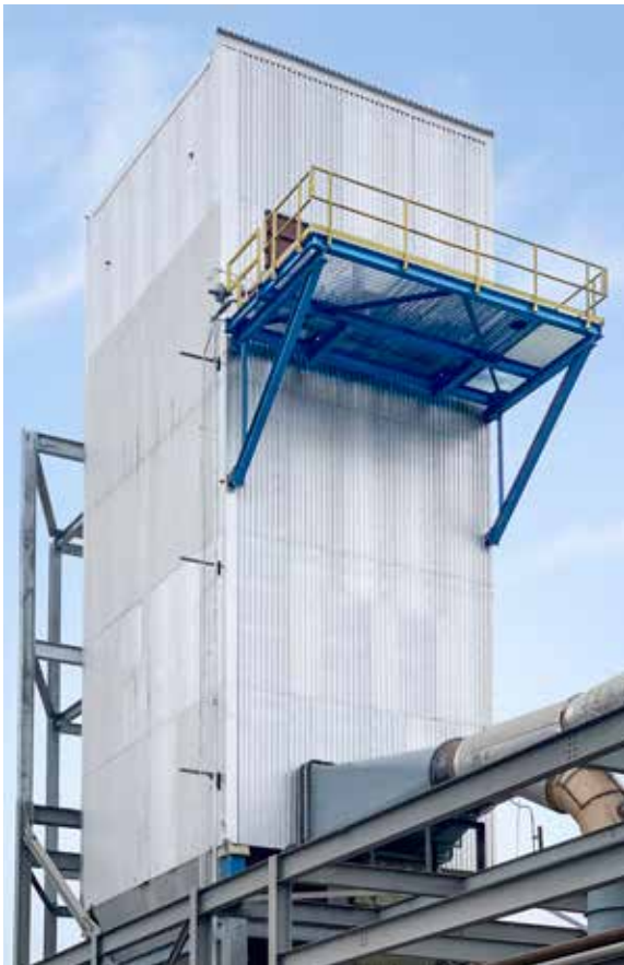
Fabric filter for particulate control
