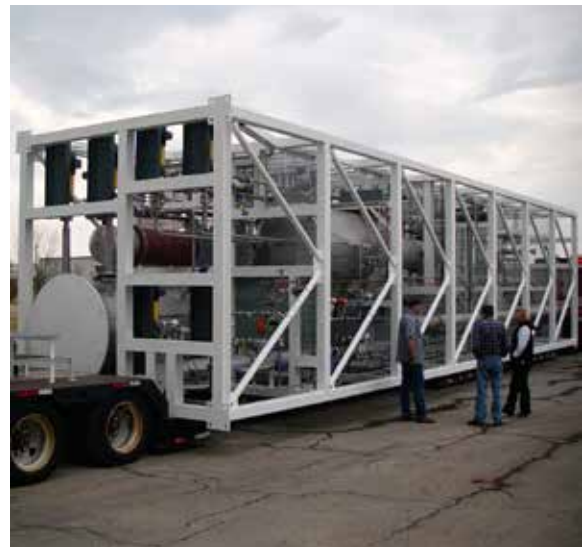
Pre-assembled distillation system on skids
