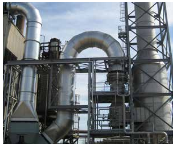
Venturi scrubber on coal-fired boiler
