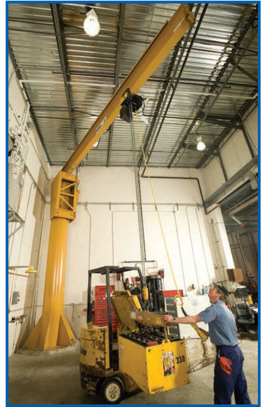
A 3-ton Spanco Freestanding Jib Crane replacing motors
