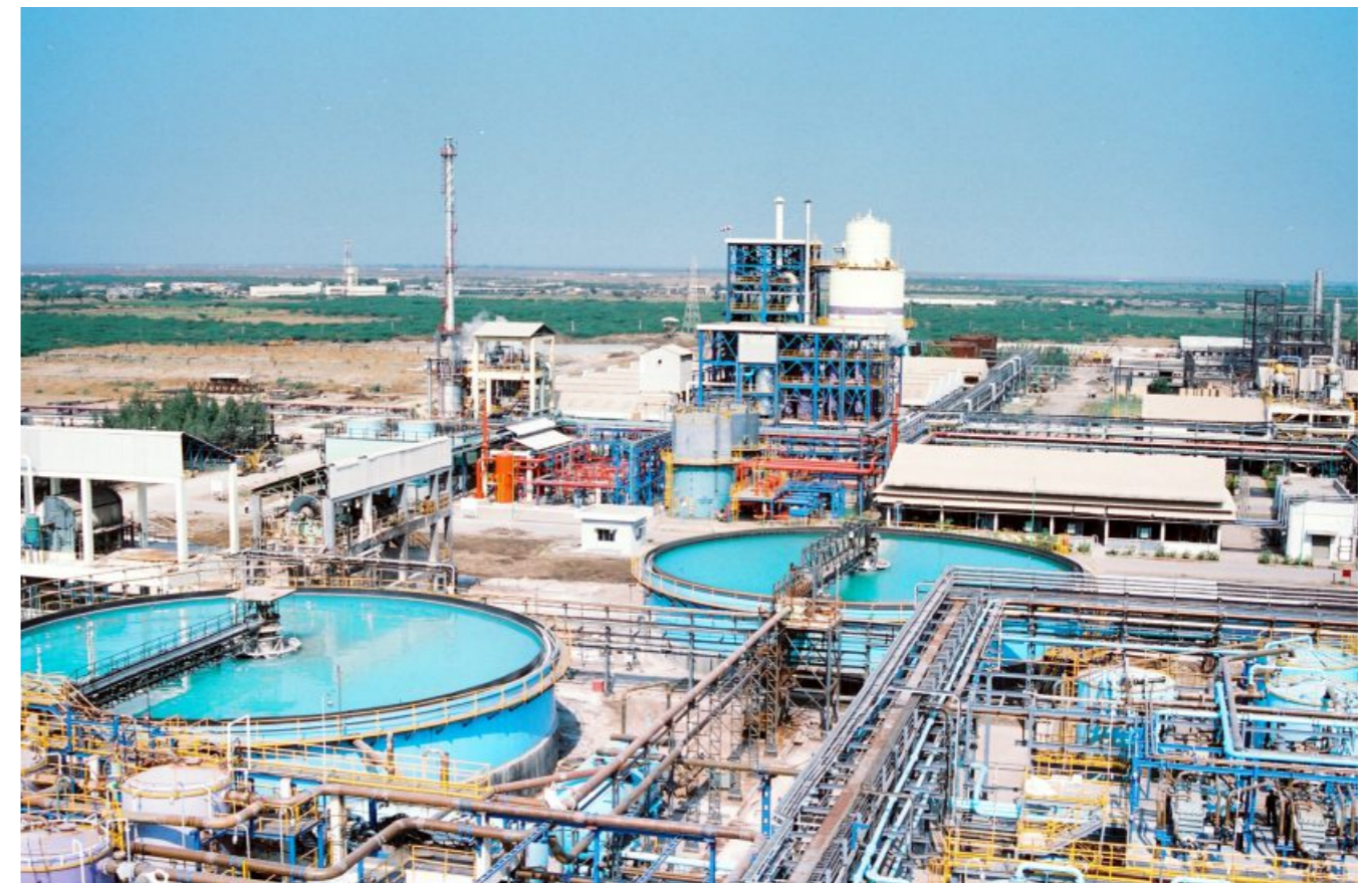
Membrane Cell Caustic Soda-Chlorine Complex
