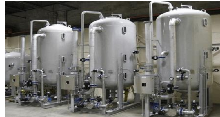
ION EXCHANGE SYSTEM
