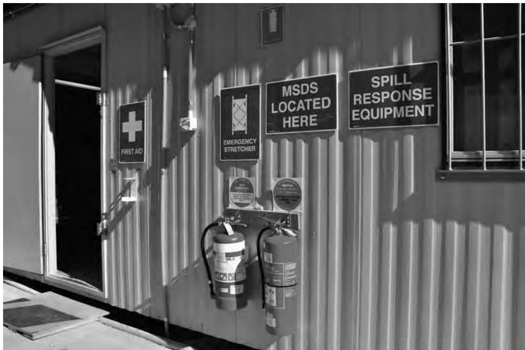
Figure 13 – First aid, fire control and emergency retrieval equipment on-site
