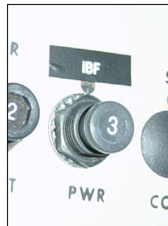
Picture 3: Circuit Breaker
