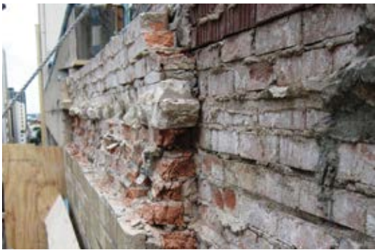
Warehouse Building deteriorated brick at parapet wall
