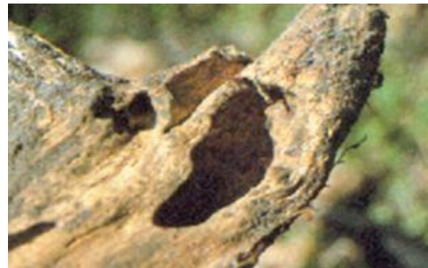
Wood damaged by Carpenter Ants.
