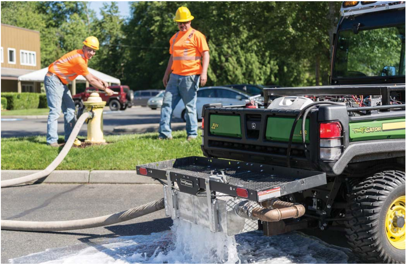
We built a custom diffuser for exercising hydrants and mounted it to the rack of the Gator. Not only is this a faster option, it is also cleaner as we can usually park over a catch basin or at least stay in the street with the water.
