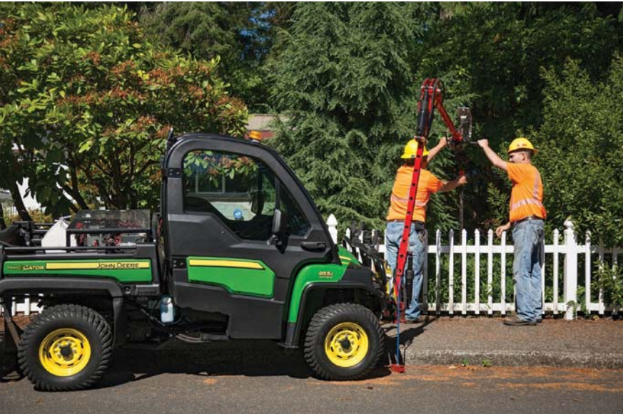
This valve is in a homeowner's nice landscape behind their fence. Without the automated turner crews would have to stand in the flowerbed to operate the valve.
