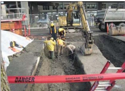
The excavator bucket is resting on a duct bank that was found to be seven feet wide. It was very heavy so required a massive support structure. In other locations, duct banks were two feet from expected locations, changing construction for shoring walls and the seawall concrete support slab. In this location, advance utility records research did not reveal the actual condition, so it became necessary to change the protect-in-place support requirements during construction.
