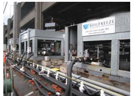
Soil freezing required several 600 amp services for chillers, as well as significant space for chillers, switchgear, and piping.
