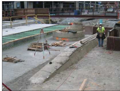
Madison Street duct bank surprise.
