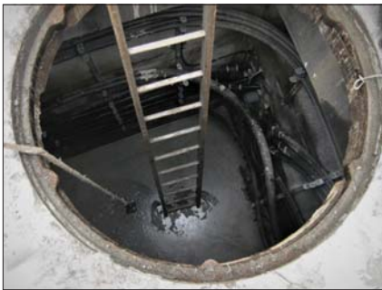
There is a foot of liquid grout in this electrical vault. Seattle City Light cleaning and repair was necessary.
