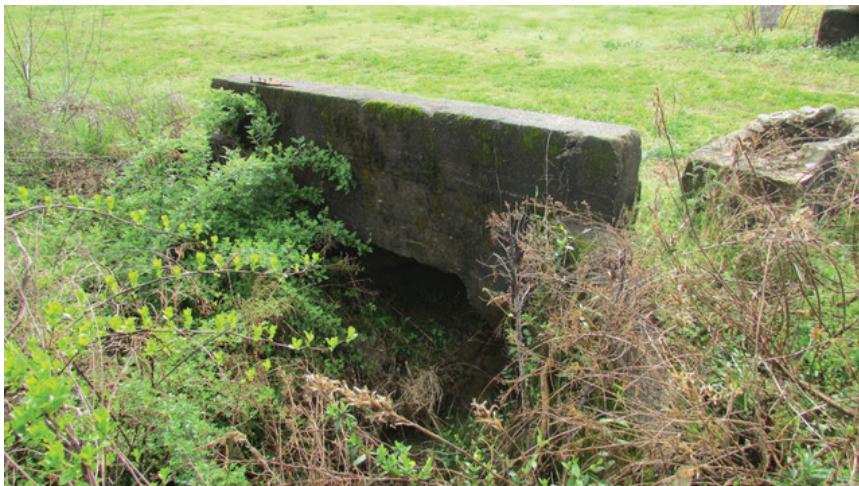
Figure 4: Detail of old bridge on original Dixie Highway. (Photo by Lamar Nelson)
