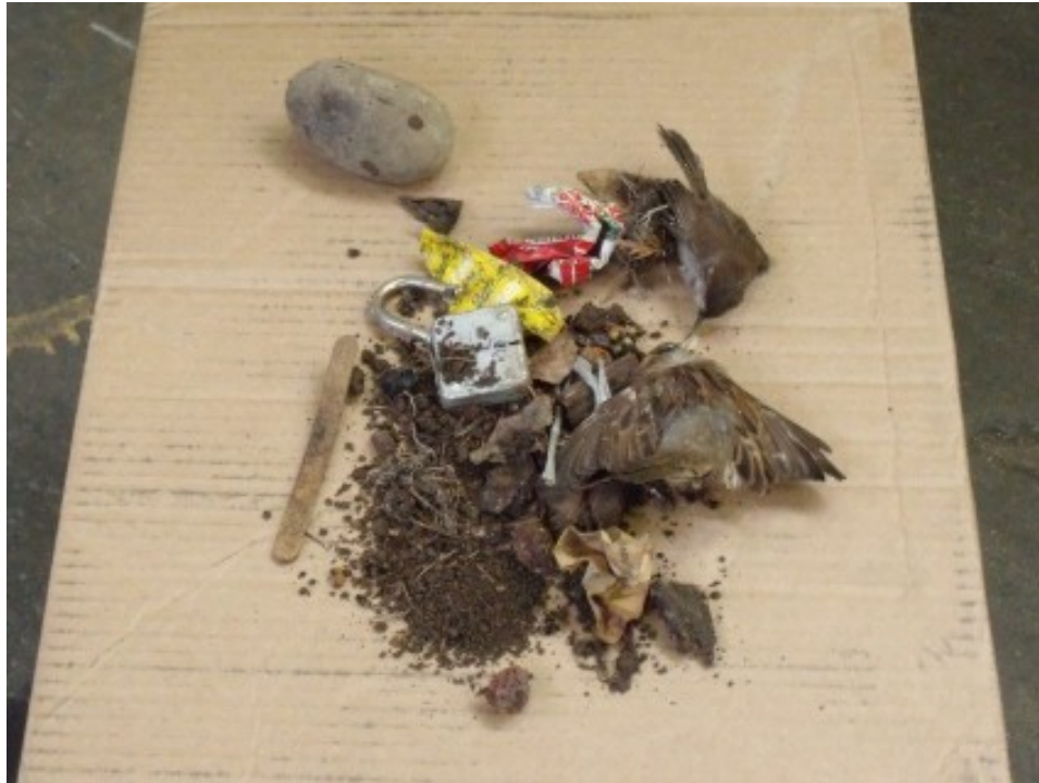
Items removed during FDC back flush
