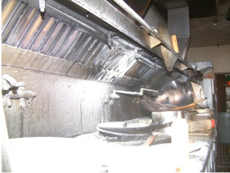
Kitchen suppression system failed to operate
