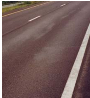
Photo 27. Bleeding of asphalt mixture.
