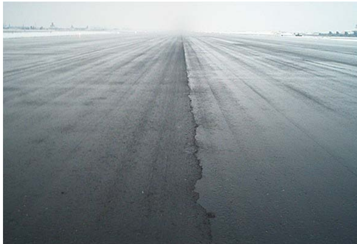
Photo 30. Cracking in joint.
