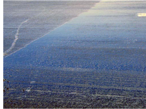
Photo 15. Excessive tack coat.
