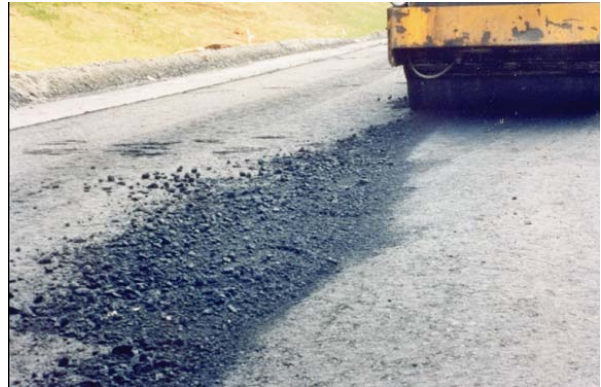
Photo 21. Segregation caused by handwork.
