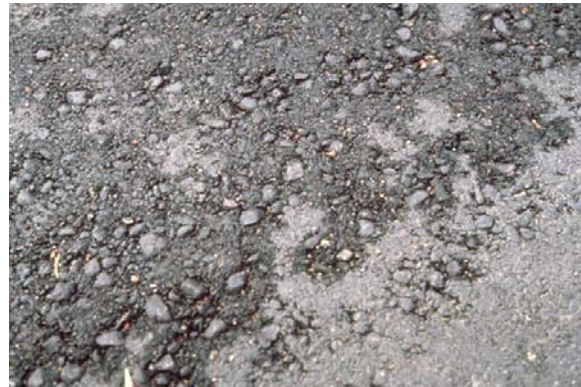
Photo 19. Segregation of asphalt concrete.
