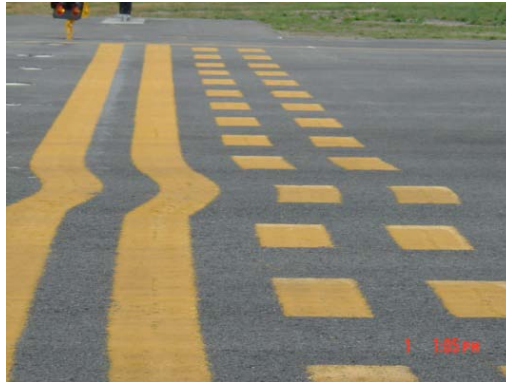
Photo 32. Slippage of asphalt mixture over underlying layer.
