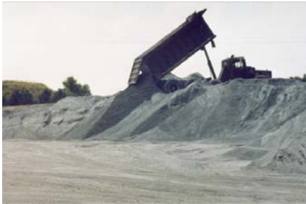
Photo 1. Improper addition of material to a stockpile.
