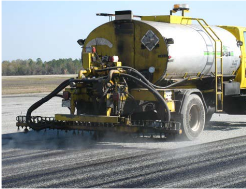
Photo 14. Asphalt distributor with uneven application.
