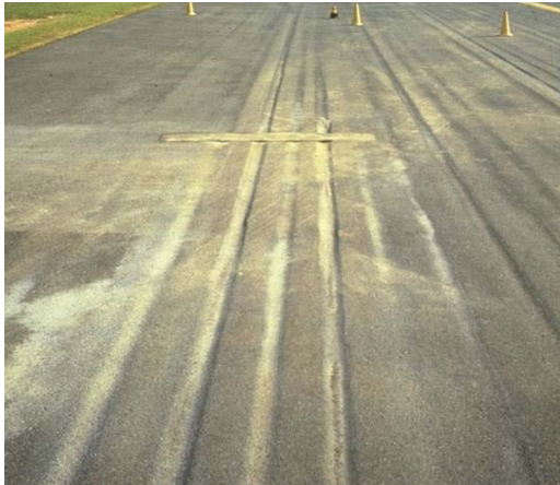
Photo 25. Rutting caused by asphalt mixture problem.
