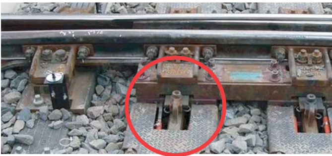
Figure E.7.2 - SwitchBlade® heater installed on frog point plates
