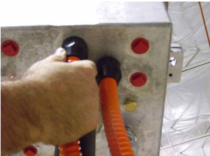
Figure D.1.7 - Direct Burial Cable Junction Box
