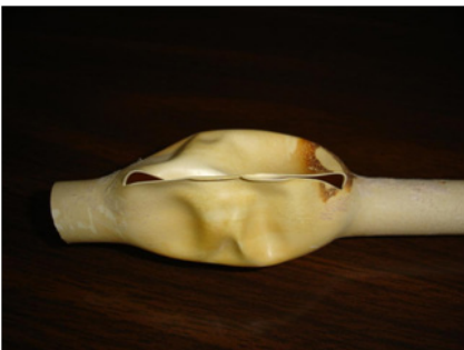
Image 24. Excessive temperature and pressure damage
