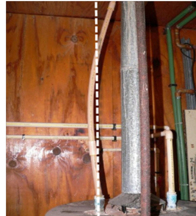
Image 12. Pipe installed near high heat
