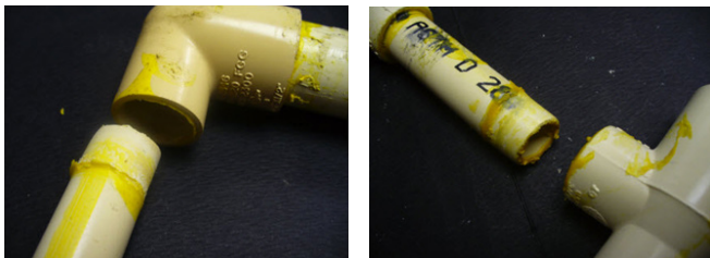
Image 22 and 23. Insufficient cement/dry joint
