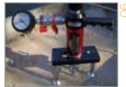
06 Conduct a pull test on each anchor using the Hydr jaws testing kit to 6kN.
