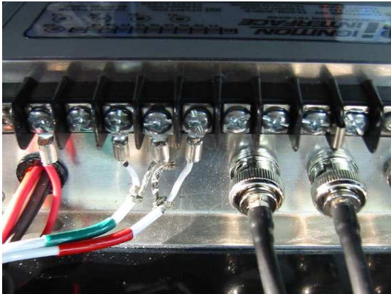
P-leads connected to G3i module.
