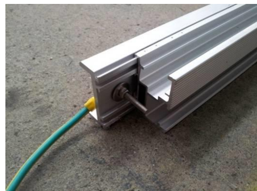
Earth cable connected to splice
