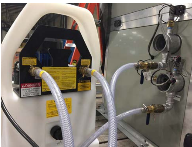
Figure 51. Rear view of Circulation pump
