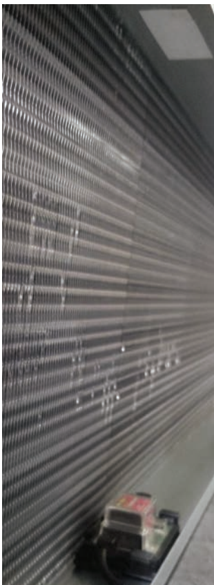
Figure 19. Moisture sensor installation and additional adhesive tape shown in cooling coil drip pan
