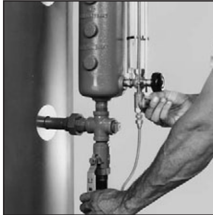
Blow down water column each morning by opening the water column and water gauge blow-off valves.
