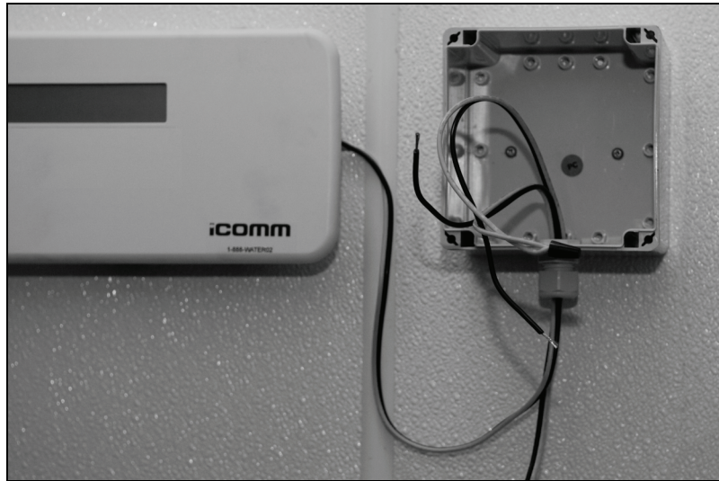
Alarm Box mounted - wiring routed inside enclosure
