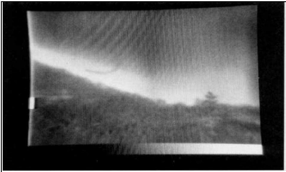
Photo 25: Site #2 - Infrared Image of Slab Edge as Viewed From Outside
