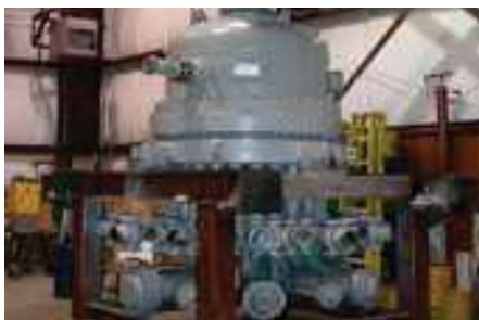
high risk of internal leakage but internal dead volumes
