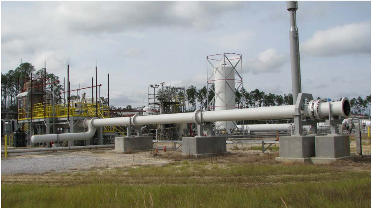
Figure 4. Photograph of the CSG Unit with Discharge Piping.
