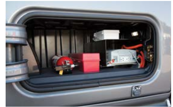
Factory-installed 1,500 watt inverter
