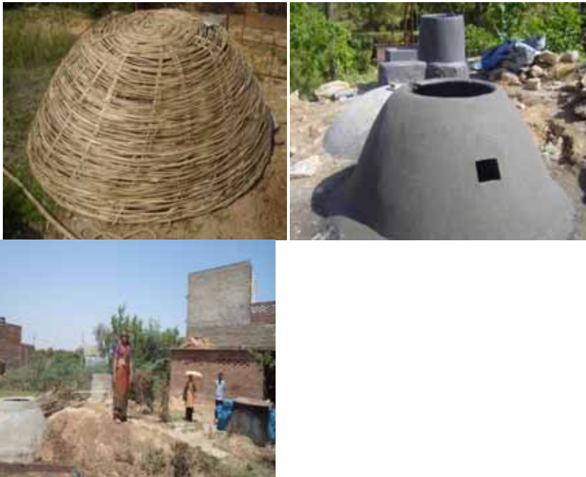
Pictures: Bamboo basket as reinforcement for cement dome for biogas, biogas plants under construction, finished biogas plant covered with soil
