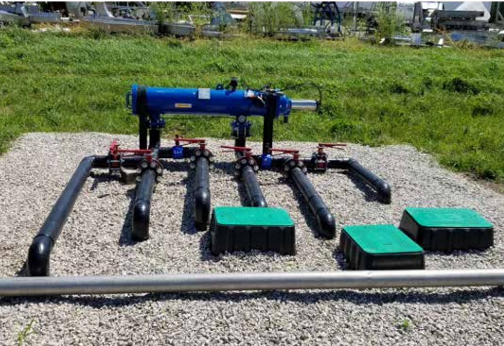
A self-cleaning filter is used at Seaquist Orchards in Door County, 2019, to remove cherry pits and pulp from water before sending it to a drip irrigation system. The manifold allows for different water sources to be filtered and transferred to multiple watering locations.
