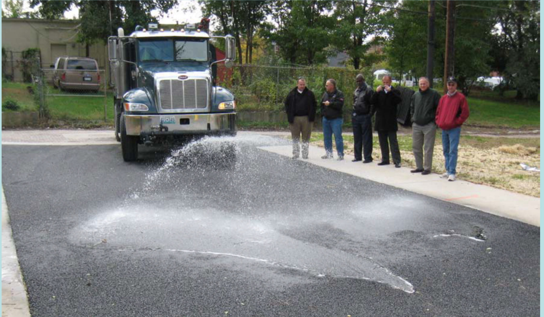
Porous asphalt alley, St. Louis, MO. Source: Metropolitan St. Louis Sewer District
